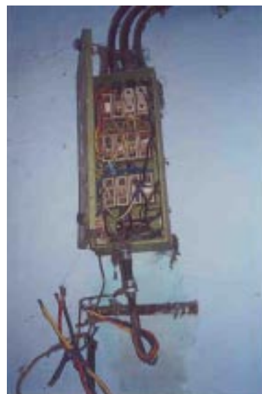
Unsafe electrical installations (Source: CLRI)
